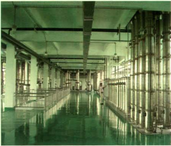
Tea bioactive compound extraction factory in Jiangsu
